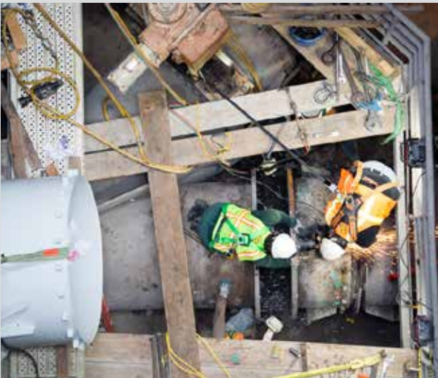
Successful installation of the new grey flange coupling adapter within Westside Pump Station Discharge Manifold Room.
