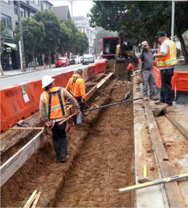
Excavation and forming for planters, Wiggle Neighborhood Green Corridor, Phase 1 - Oak & Fell Streets/Channel GI
