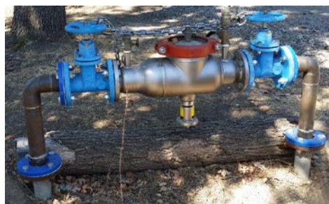
Example of a backflow prevention assembly
