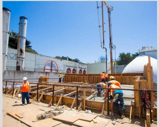
OSP Flare Controls and Stack Upgrade: placing concrete roof slab for new bldg 821
