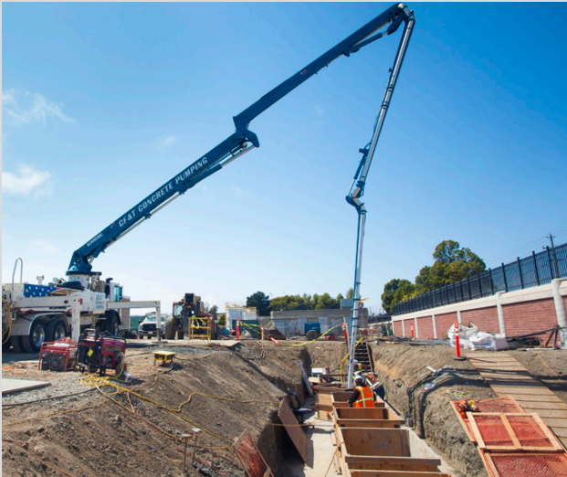
SEP 521/522 and Disinfection Upgrades Projects: Concrete placement for the new No. 3 water pump trough inside the Chlorine Contact Channel
