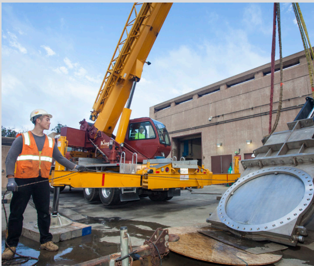
Westside Pump Station Reliability Improvements Project: Removal of existing 54-inch Flange Coupling Adapter and installation of new 54-inch Knife Gate Valve on the discharge pipe manifold
